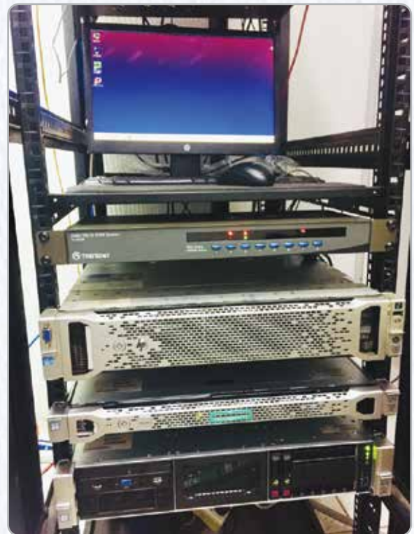
Upgraded Server Room at Head Office.
